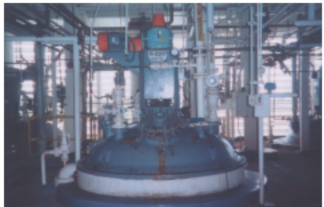
4000 Gallon Pfaudler Glass Lined Reactor In Plant 2
