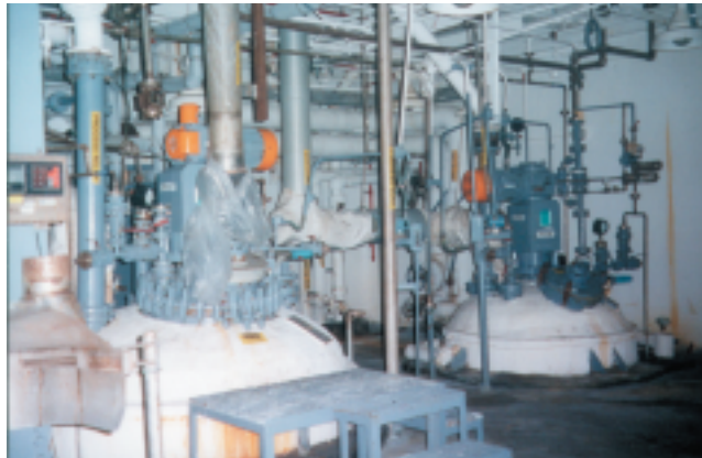
A Bank Of Glass Lined Reactors In Plant 1
