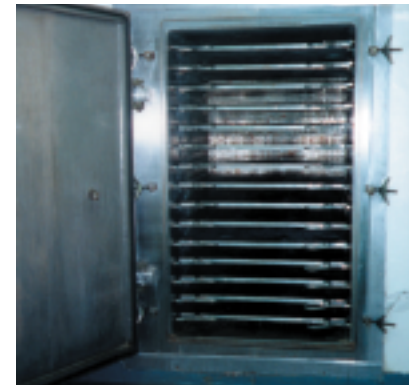
1 Of 3 Shelf Dryers In Plant 1
